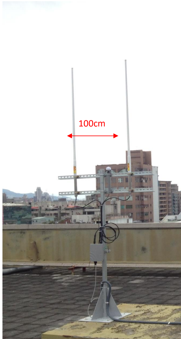
Figure 33 Actual View of a Base-mount Installation
