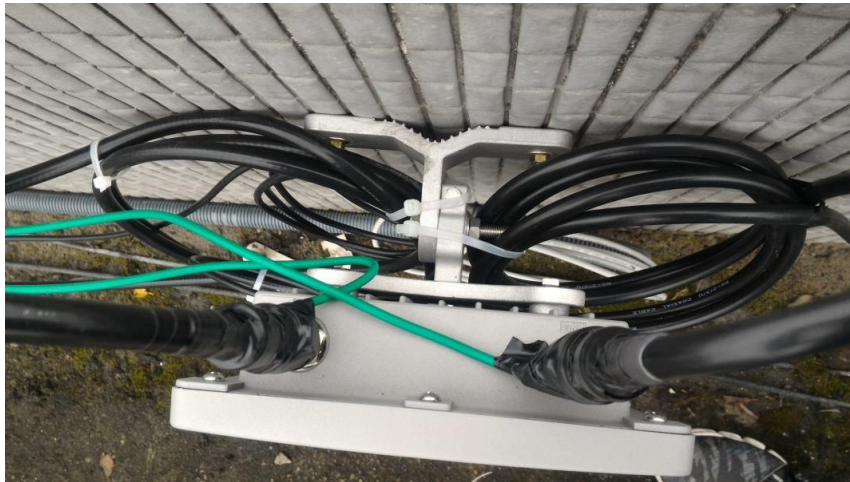
Figure 30 Lightning Protections and Grounding Equipment – Image 1
