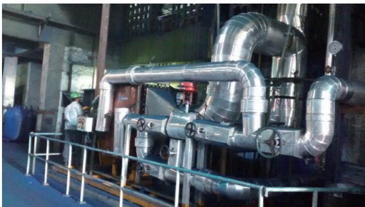
Industrial Heating Equipment
