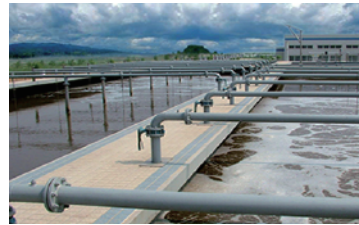
General Water Treatment
