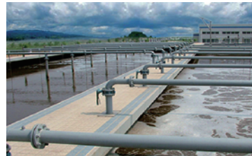
General Water Treatment
