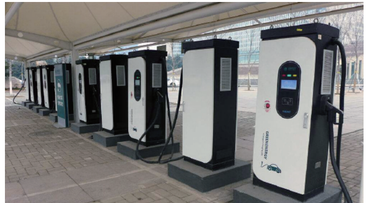
Car Charging Pile
