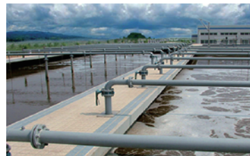
General Water Treatment
